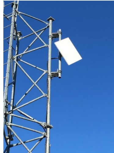
Figure 2. MWRA Microwave Antenna
